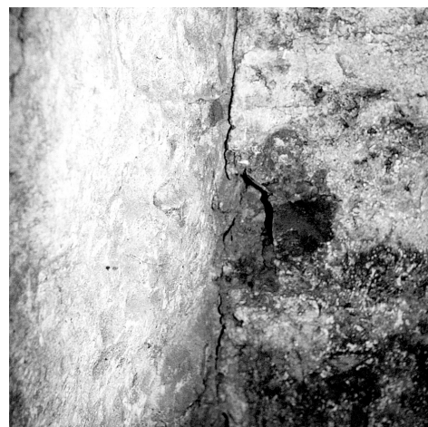
234 Thun, Obere Hauptgasse 35, Detail Baunaht (Riss), Foto 1999.
