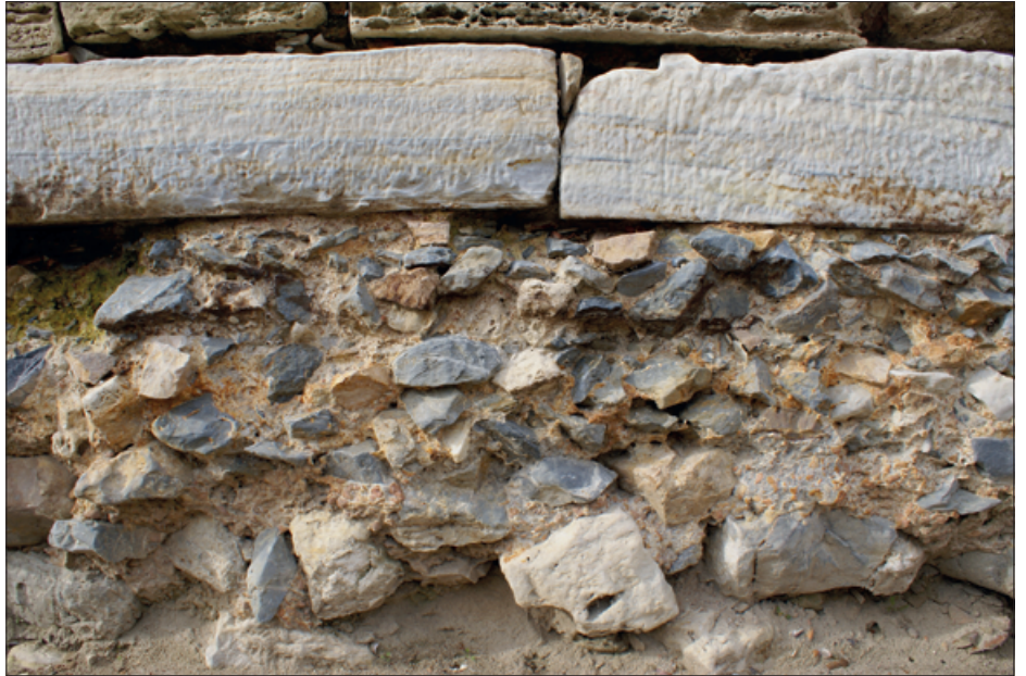
Fig. 7 Yenikapı, concrete filling of the wooden formwork. – (Photograph A. Ercan, from Ercan, Yenikapı 122, detail).
