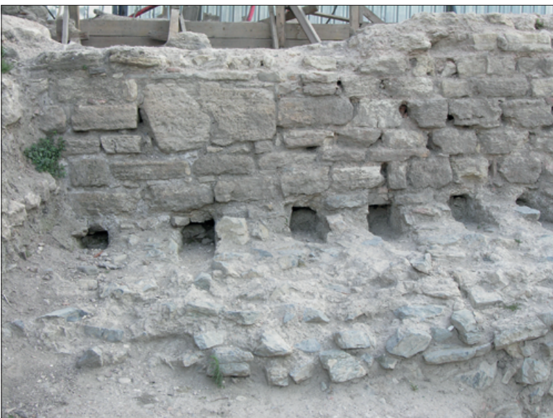
Fig. 32 Yenikapı, row of holes for wooden beams. – (Photograph B. Köşker, IAM Archive, from Gökçay, Architectural Finds 171).
