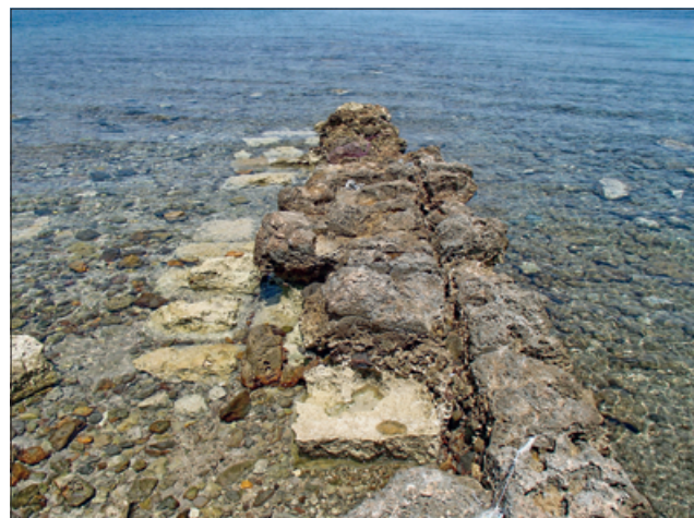
Fig. 21 Detail views of the eastern mole construction of the harbour of Anthedon. – (Photo A. Ginalis, 2018).
