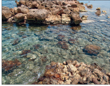
Fig. 19 Breach of the northern mole construction of the harbour of Anthedon. – (Photo A. Ginalis, 2018).
