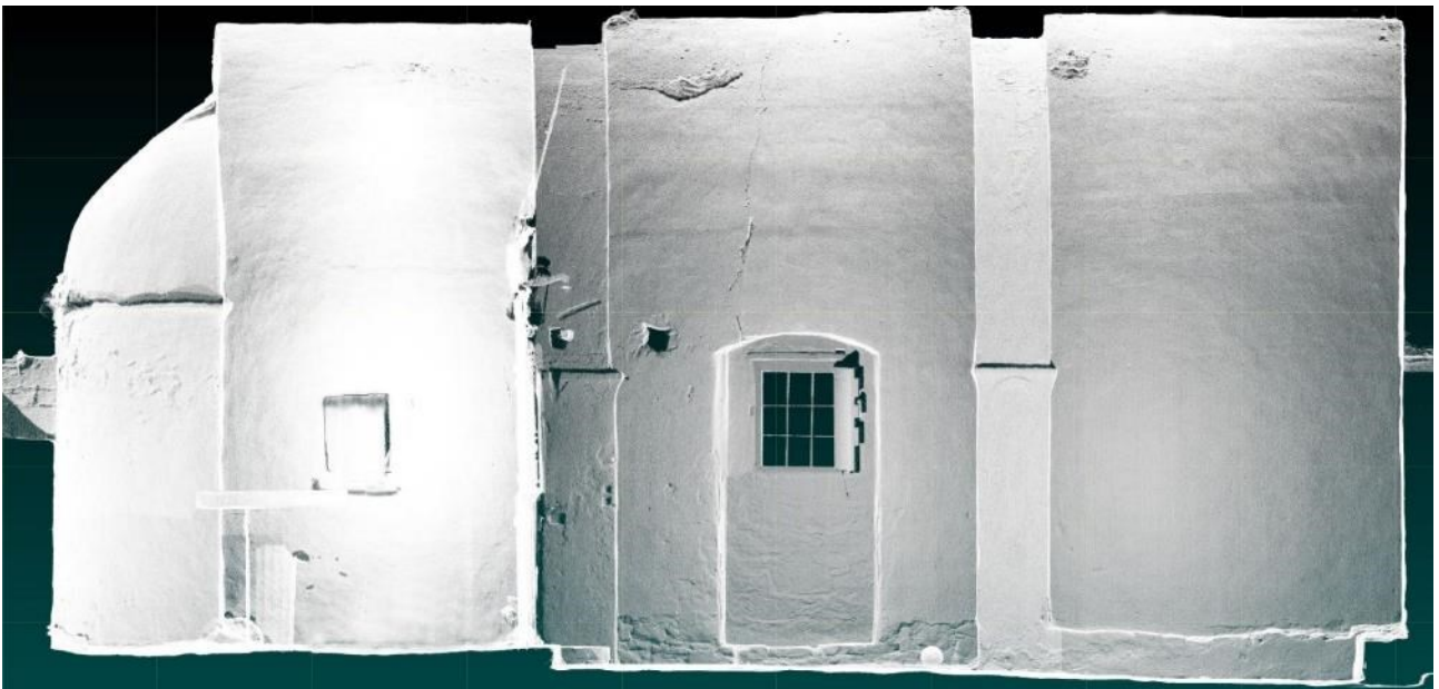
Fig. 5. Orthophoto of the north facade of St Ioannis Prodromos Church in Axos, without RGB filters, used for crack detection.
