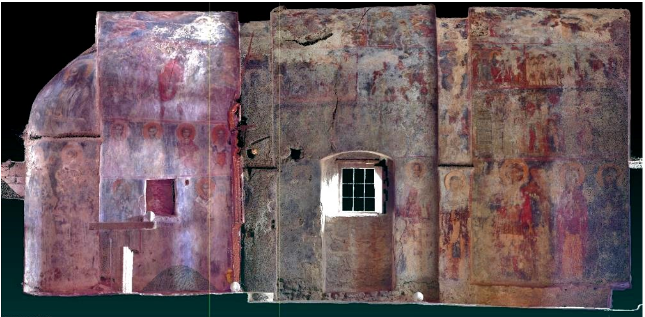
Fig. 4. Orthophoto of the north facade of St Ioannis Prodromos Church in Axos.
