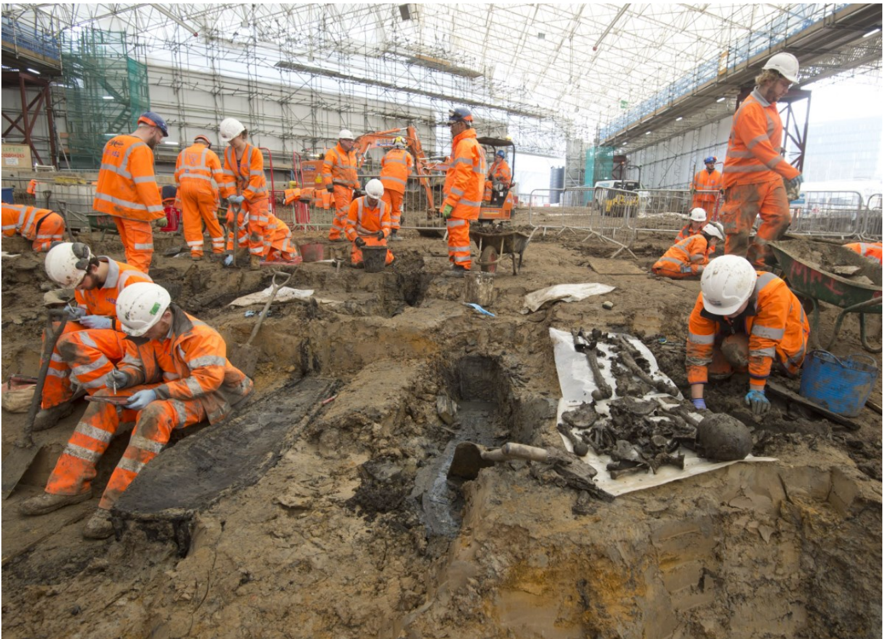
Fig. 2. Archaeologists excavating the St James Burial ground for HS2 (© HS2) courtesy of MOLA Headland Infrastructure.
