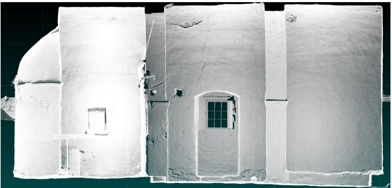
Fig. 5. Orthophoto of the north facade of St Ioannis Prodromos Church in Axos, without RGB filters, used for crack detection.
