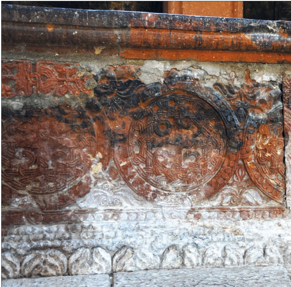
Fig. 17 Marmashen Monastery, main church (1029): fragment of the wall of the altar's elevation. – (Photo A. Kazaryan / L. Mikayelyan).
