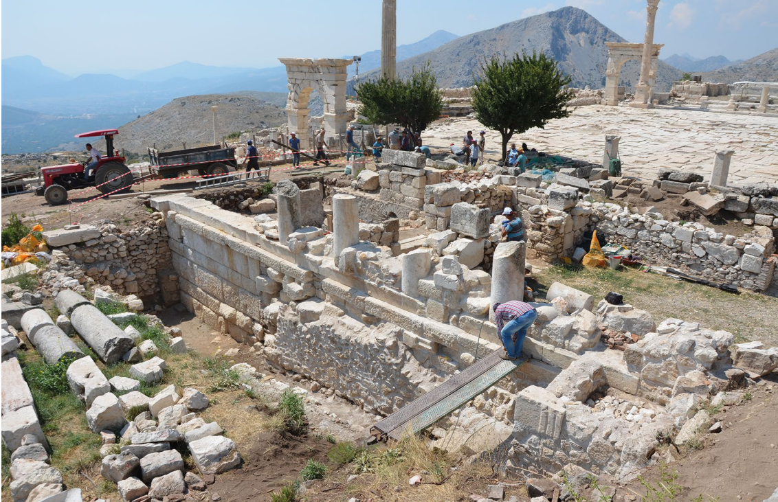
Fig. 2: Remains of the middle Hellenistic Market Building(?) under excavation and conservation at Sagalassos. Remains of the original building formed part of series of transformations into late antiquity.
