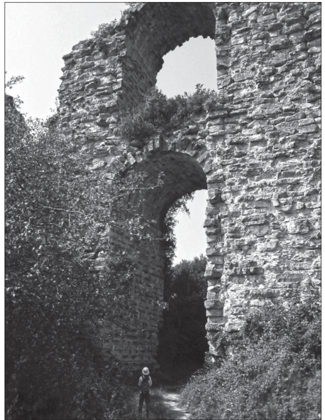
Fig. 7 5 th century aqueduct bridge of Kumarlıdere with exposed mortar and rubble core. – (Photo R. Snyder).
