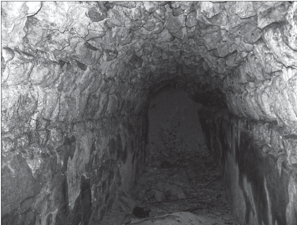
Fig. 5 Small section of intact channel near Binkilic showing arched limestone vaulting and channel lining mortar of the channel walls and floor. – (Photo J. Crow).
