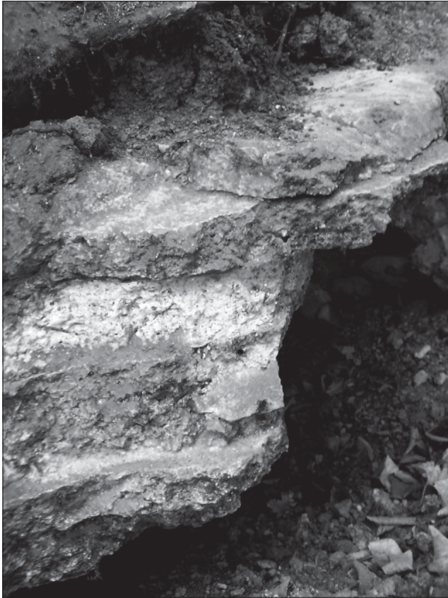
Fig. 10 Channel lining mortar in situ showing multiple events of re-plastering. – (Photo R. Snyder).
