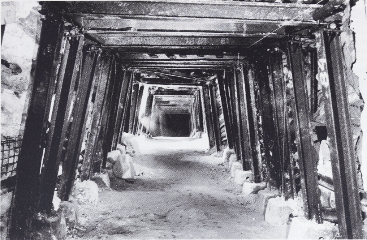
Fig. 12 The modern tunnel dug right across the prehistoric mining area after having been secured with steel supporting props.
