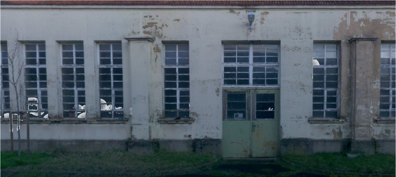
Fig. 1. A part of the façade of “Halle 6” that was the focus of our study (© Authors).
