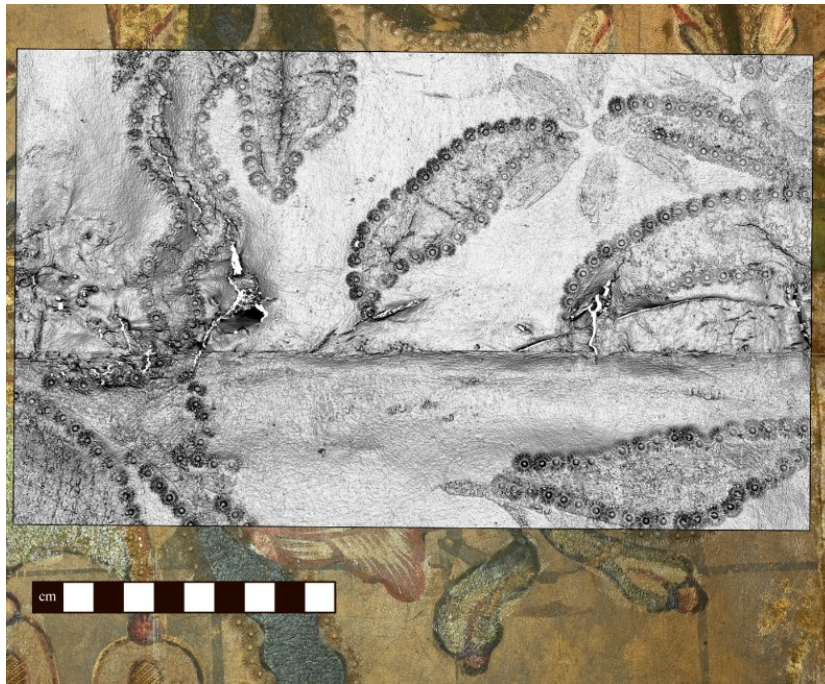
Fig. 2. Reference area of the leather panel in the Chinese Room in Moritzburg Castle taken by the SLS and laid on top of an orthogonal colour photograph. The grazing light increases the visibility of cracks and losses along the seed of two leather parts (© Leander Pallas).
