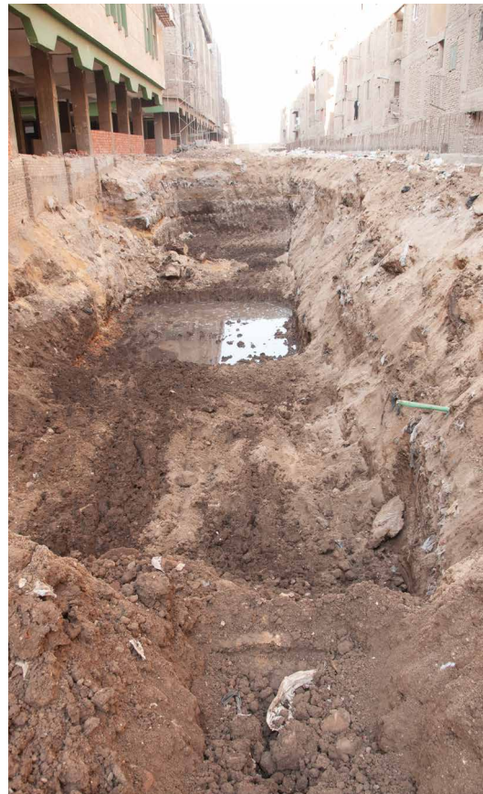
Fig. 5: Area 203 (view into the construction trench of new buildings; spring 2015); shopping mall (left) and residential houses (right); Photo: D. Raue.
