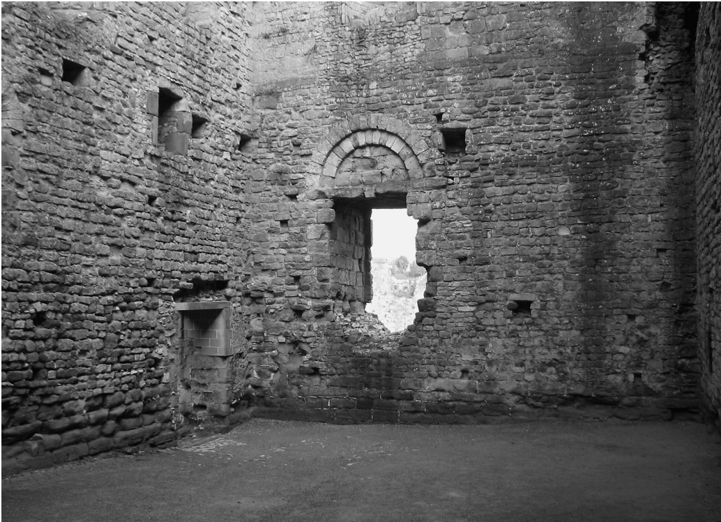
Abb. 8 The interior of the east wall of the great tower at Chepstow seen from ground level. The arched doorway, with a decorated tympanum on its external face, was probably the principal entrance to the tower, though it opens into the basement. Though altered, the door to the left at ground floor level appears to be an original eleventh-century feature (Matthew J. Strickland).
