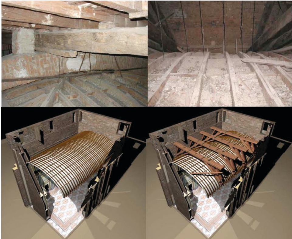
Fig. 12 Above, images of the extrados of the wooden vault of the Ballroom. Below, 3D model of the vault.
