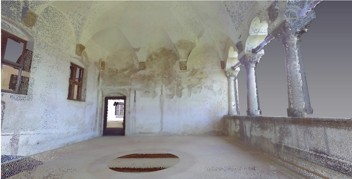
Fig. 39 Internal view of the loggia; high point density gives detailed representation of individual features.
