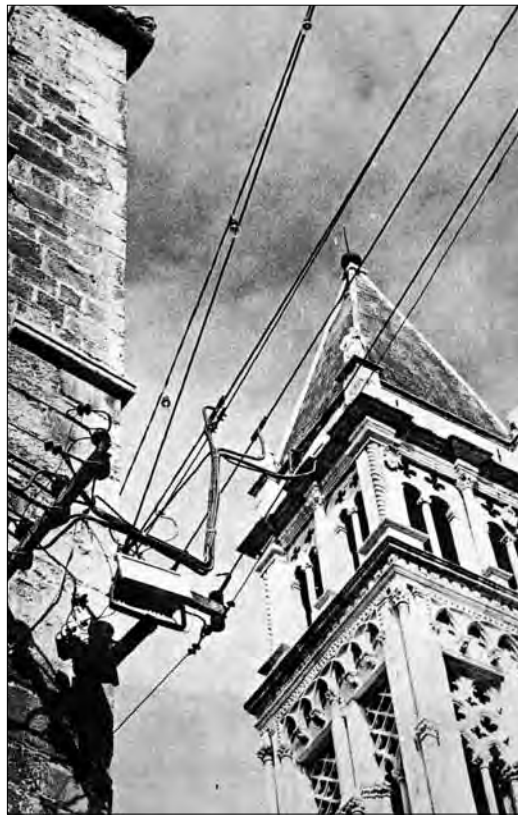
Fig. 3: Nada Orel, Electrical installations in the centre of Trogir, 1976, published in Arhitektura 160–161/1977, 5
