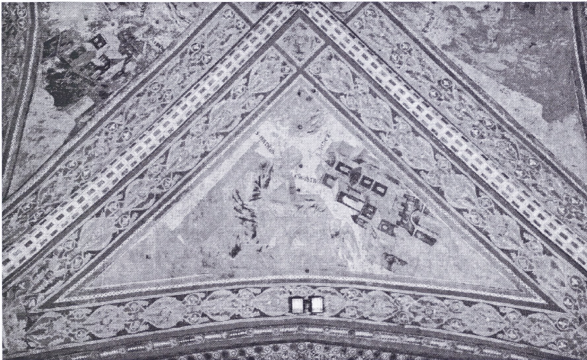
Fig. 1: The S. Matthew fresco, painted by Cimabue for the Upper Church of S. Francis in Assisi. The fresco, having an extension of 35 squared meters, has been broken into more than 120.000 pieces by the earthquake in September 1997.
