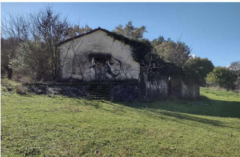
Fig. 4: Building in decay, Ziros Children's Town, Greece
