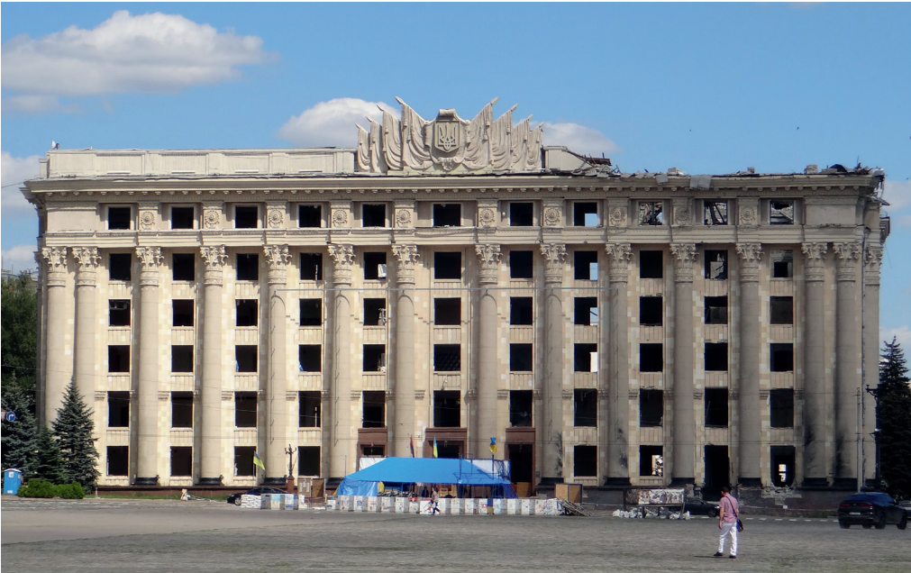
Fig. 19 The building of Kharkiv Regional State Administration on Sumska Street, 64. June 2022. Photo Svitlana Smolenska.
