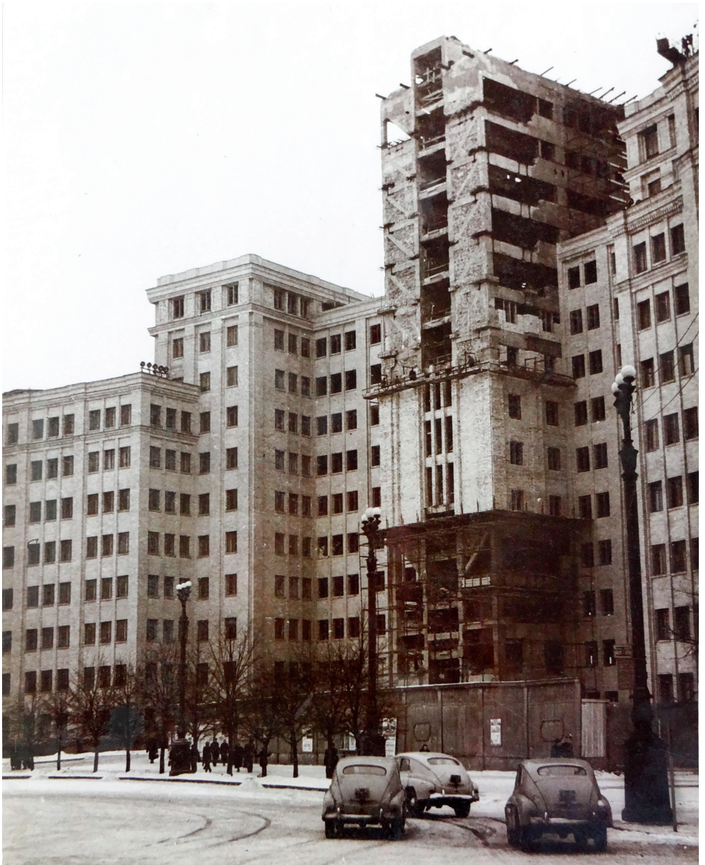
Fig. 8 V. N. Karazin Kharkiv National University (The House of Projects) during the reconstruction period. Photo 1959 © The archives of V. N. Karazin Kharkiv National University library.
