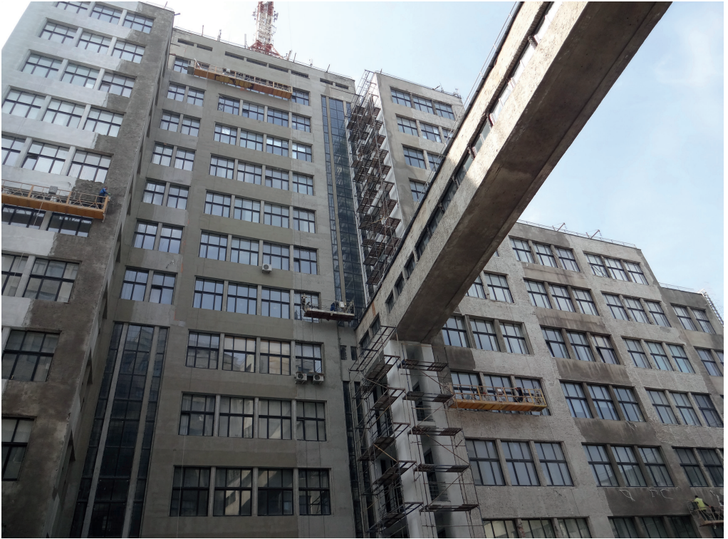
Fig. 15 Facades of Derzhprom in the process of their repair, state 2014. Photo Svitlana Smolenska.
