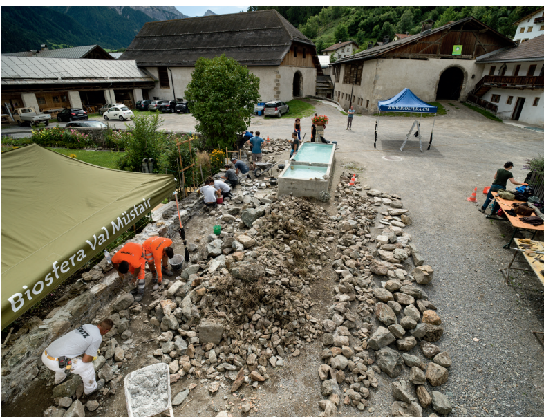
Fig. 4: Masonry workshop in the western courtyard of the convent of St. John, Müstair (2020).
